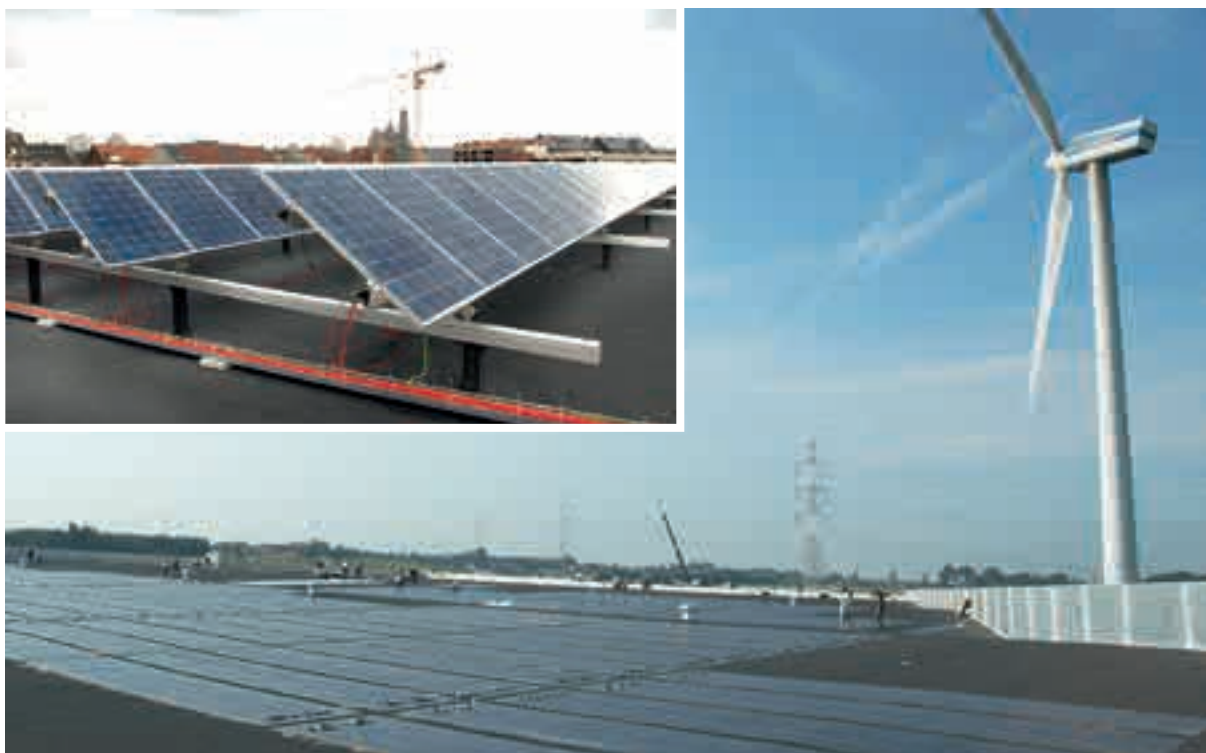
The solar panels on the roof of the store in Ninove and the distribution centre Dassenveld in Halle
