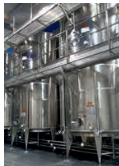
The brand-new stainless barrels in the wine cellar in Ghislenghien
